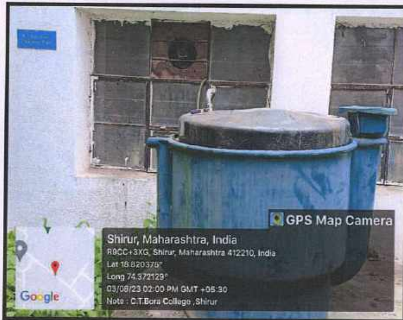
* Photograph of Kitchen Waste treatment plant near Ladies hostel kitchen
